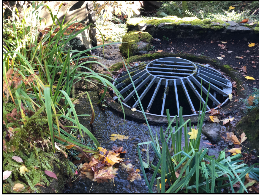
View of catch basin looking east. Note water flowing through a break in the wall around the catch basin.
